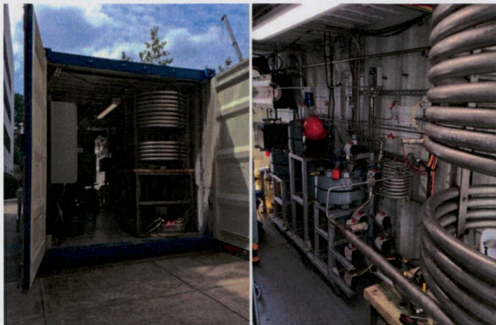
Figure 2. Duke SCWO pilot-scale system (during construction, thermal insulation removed). The system is housed in a standard 20 ft shipping container and can treat about 1 ton (or 270 gallons) of waste per day.
