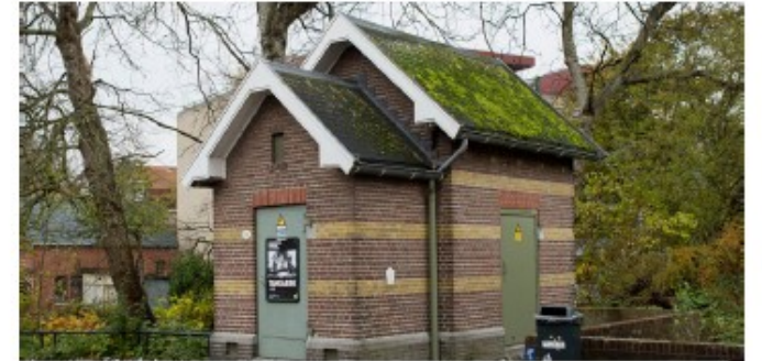
MS-MS station (3-23kV)
